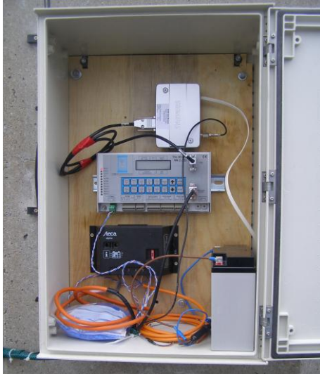
Fig. 2a: Data logger with Wi-Fi Modem and power supply using battery
